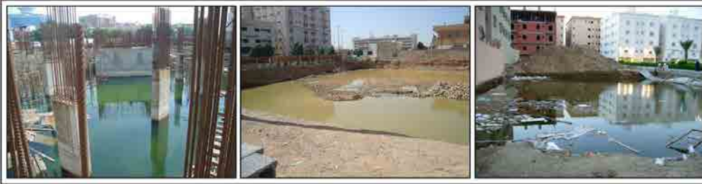
Figure 5. Housing constructions that had earthworks done and so formed environments for mosquitoes to breed (photos: H.Khormi).
